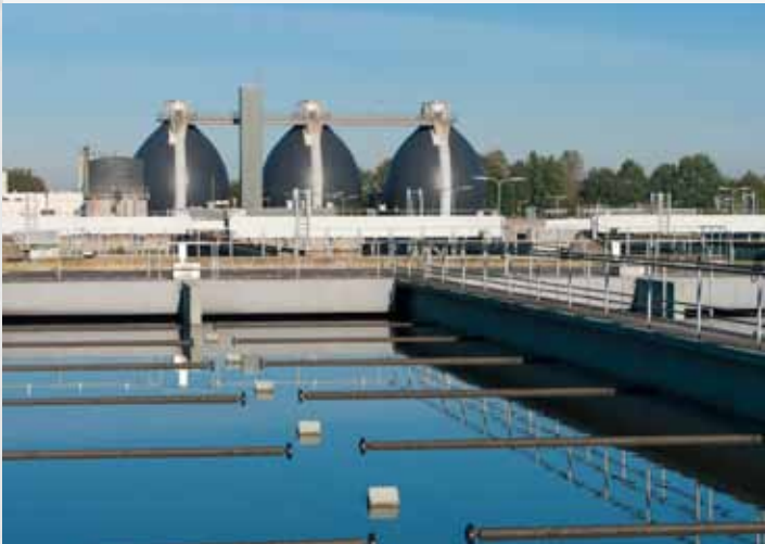
Waste water treatment facilities
