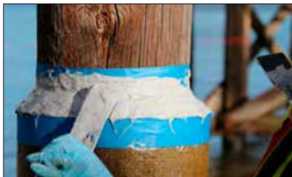
Install FX-763 Trowel Grade Epoxy at the head of the jacket and finish to a 45° tapered bevel, creating a water and chemical-resistant barrier to the repair system.
