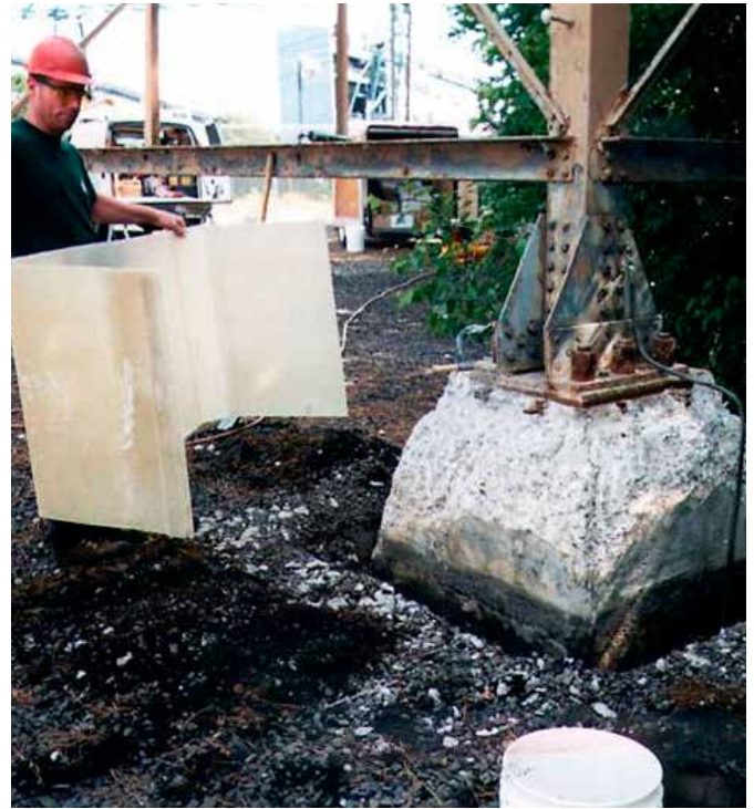
Foundation prepared and excavated; FX-70® jacket installed below ground level for additional protection
