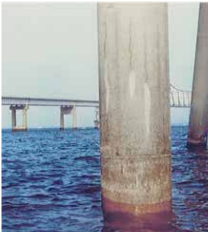
Example of pile "scour"
