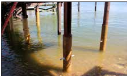
Piles with ≤ 25% section loss, fill remaining void in jacket with FX-70-6MP™. Piles with > 25% section loss, fill void with FX-225 Underwater Grout, leaving 100 mm open at top of jacket (allow to cure overnight); fill remaining 100 mm with FX-70-6MP™ (allow to cure overnight).
