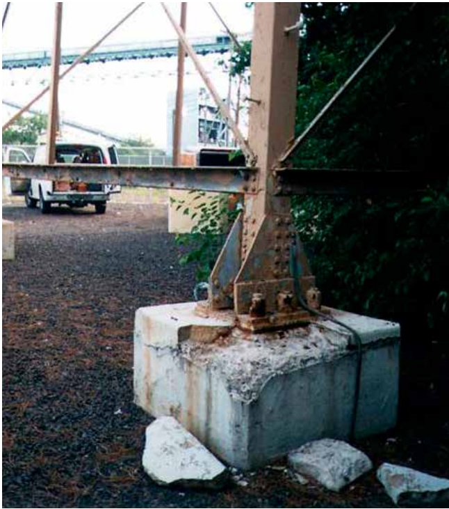
Severe damage to concrete foundation
