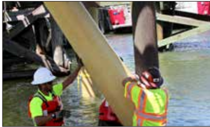
Insert the tongue into the locking groove of the jacket and position it leaving 460-610 mm of undamaged pile above and below the damaged area.
