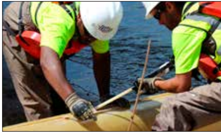
Install a bead of FX-763 into the locking groove of the jacket and place FX-70® jacket around the pile to be repaired.
